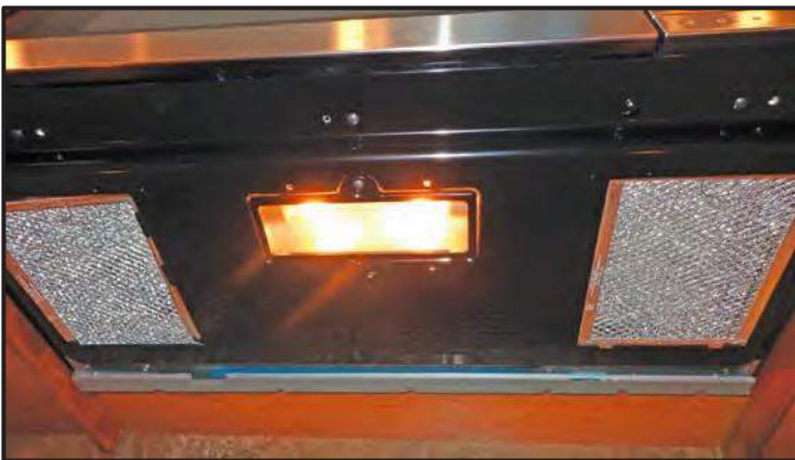
Figure 5-5: Air Filtration Fan
