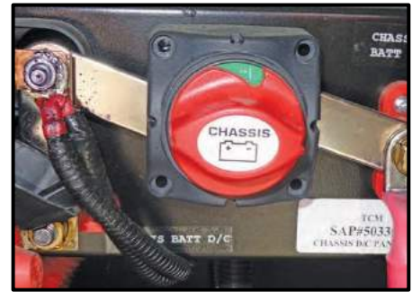
Figure 9-15: Engine Battery Disconnect Switch
