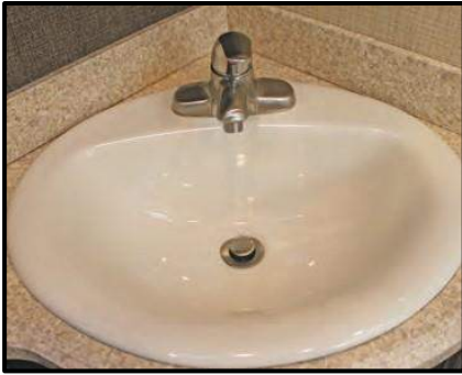
Figure 13-3: Bathroom Sink and Faucet
