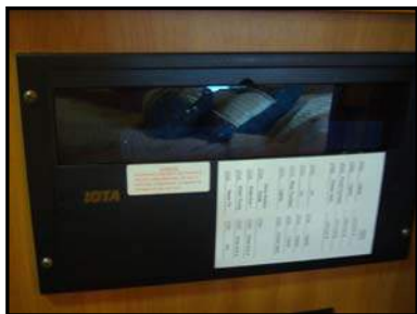
Figure 7-1. Circuit Breaker Box
