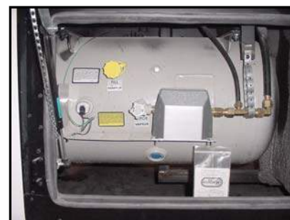
Figure 3-4. Liquid Propane Tank
