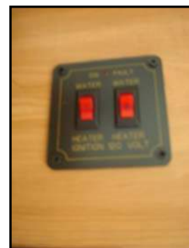
Figure 4-15. Water Heater Switches
