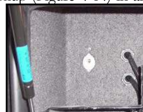
Figure 4-14. Cable & Telephone Jack
