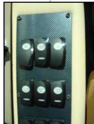
Figure 7-8. 12 VDC Disconnect Switch
