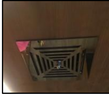
Figure 3-3: Return Air Vent
