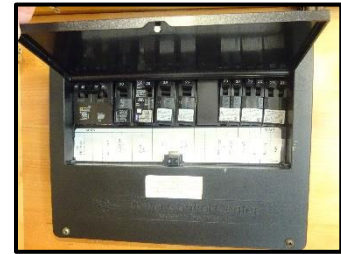
Figure 9-3: Circuit Breaker Boxes
