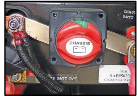
Figure 9-15: Engine Battery Disconnect Switch
