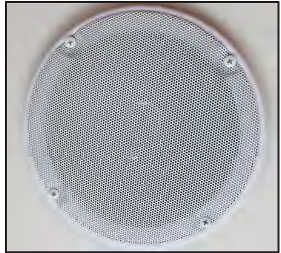
Figure 6-8: Overhead Surround Sound Speaker
