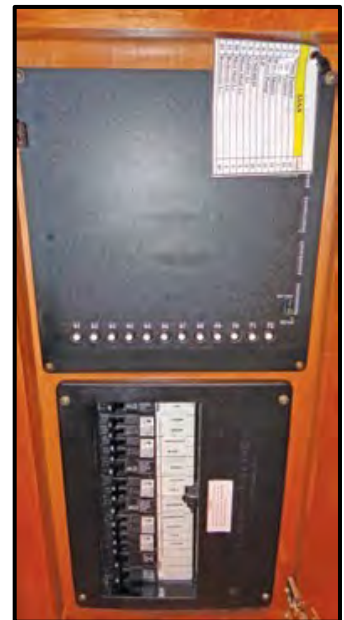
Figure 9-4: Circuit Breaker Boxes
