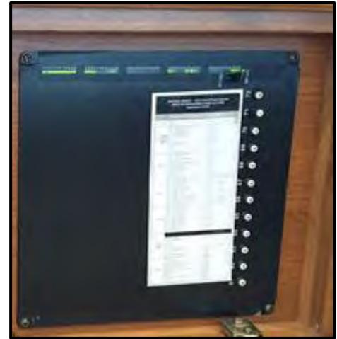
Figure 9-3: Multiplex System Switch Panel
