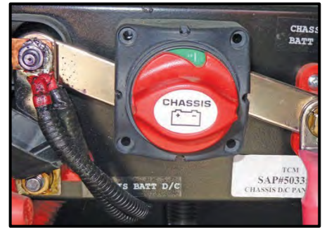
Figure 9-16: Engine Battery Disconnect Switch
