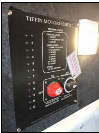
Figure 9-15: House Battery Disconnect Panel
