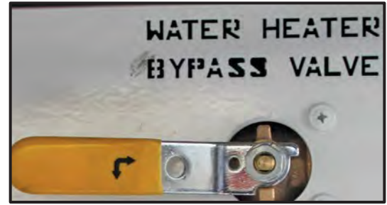
Figure 13-9: Water Heater Bypass System
