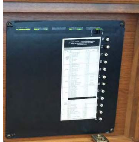
Figure 9-3: Multiplex System Switch panel
