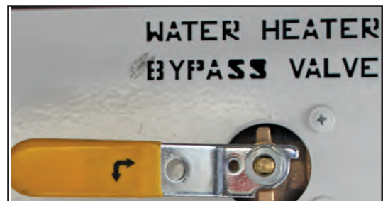
Figure 13-9: Water heater bypass valve
