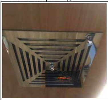
Figure 3-2: Outgoing air vent
