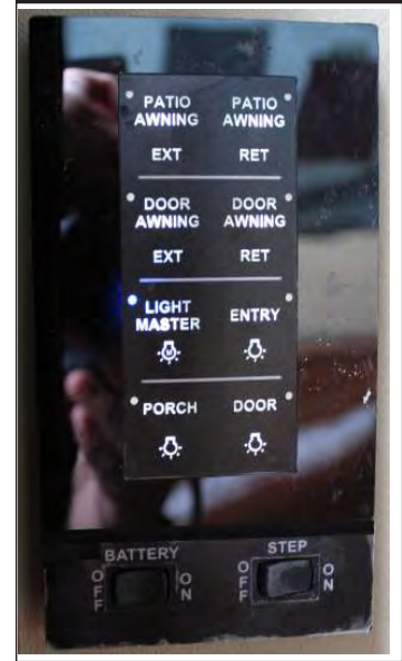
Figure 9-17: 12 VDC disconnect switch
