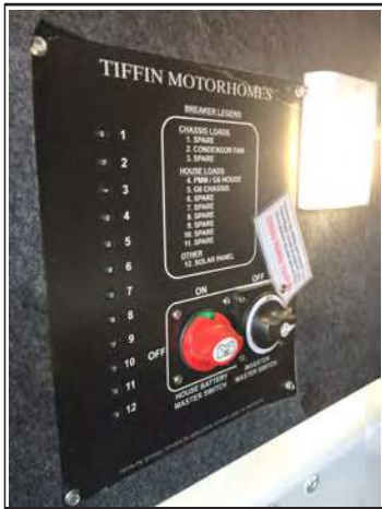
Figure 9-15: House battery disconnect switch
