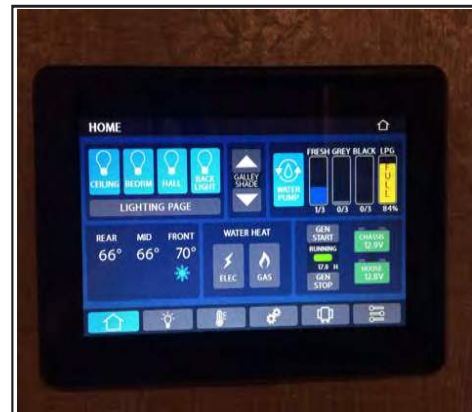
Figure 13-5: Water pump switch
