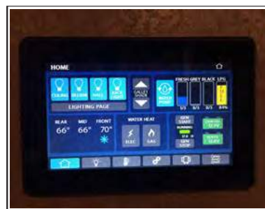
Figure 5-7: Water heater screen (Spyder control system)
