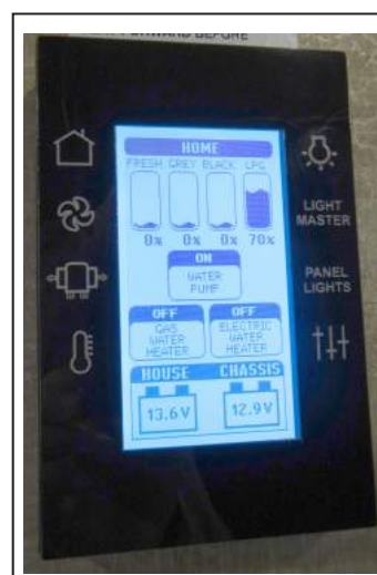
Figure 5-7: Water heater screen - Spyder control system
