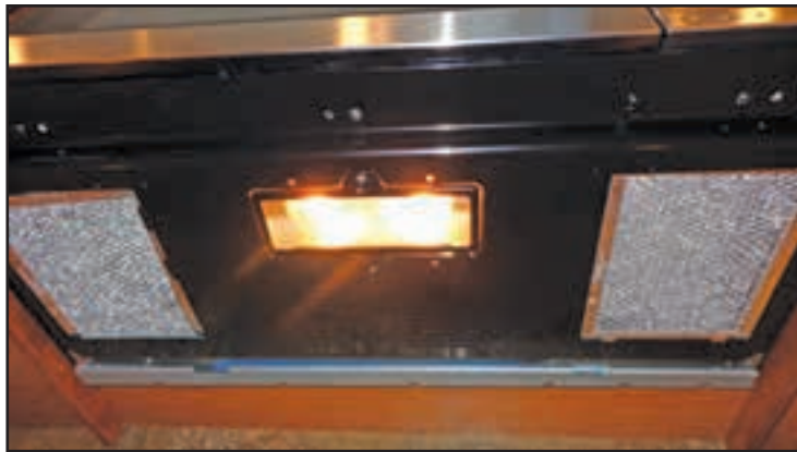
Figure 5-5: Air filtration fans
