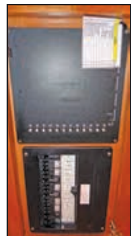
Figure 9-1: Circuit breaker box
