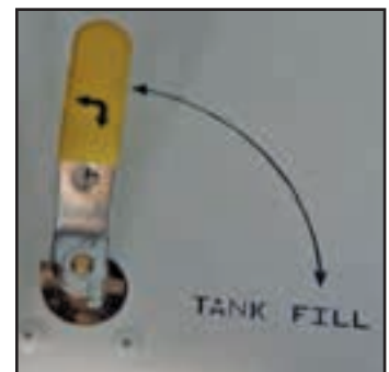
Figure 13-7: Tank fill valve
