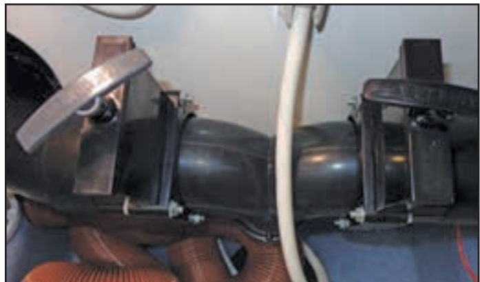
Figure 13-11: Sanitation coupling, valve and hose
