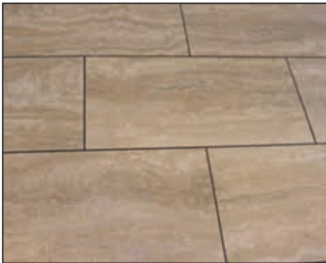
Figure 12-2: Typical flooring in the Allegro RED
