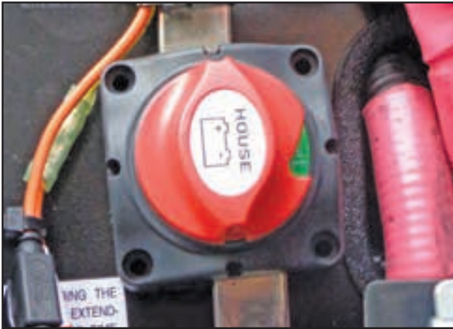
Figure 9-10: House battery disconnect switch
