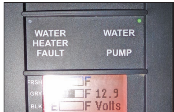
Figure 13-5: Water pump switch
