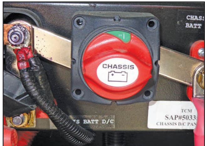
Figure 9-11: Engine battery disconnect switch
