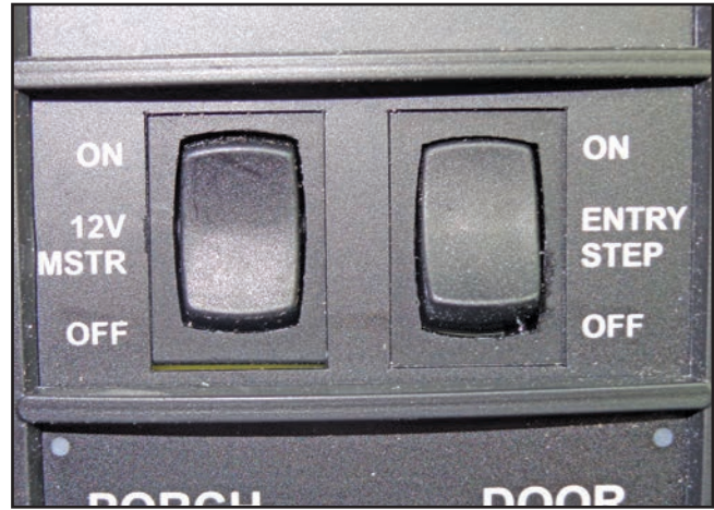
Figure 9-12: 12 VDC disconnect switch
