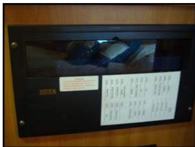
Figure 7-1. Circuit Breaker Box
