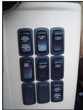
Figure 7-8. 12 VDC Disconnect Switch
