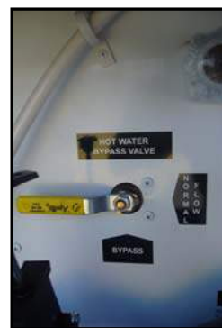
Figure 11-9. Water Heater Bypass System
