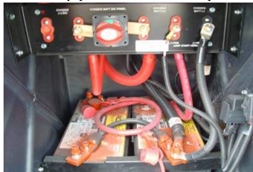
Figure 7-5. 12 VDC Battery System
