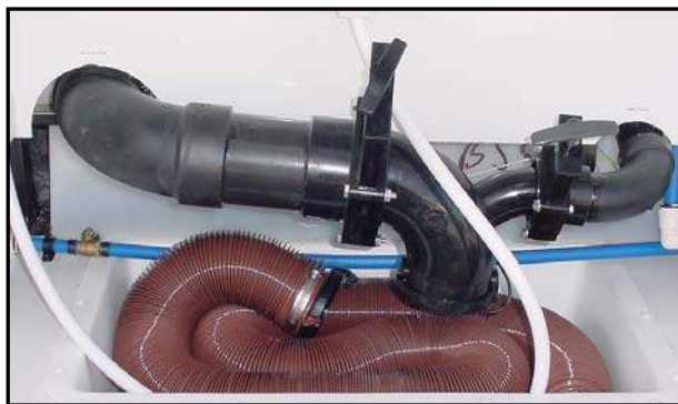
Figure 11-11. Sanitation Coupling, Valve, and Hose
