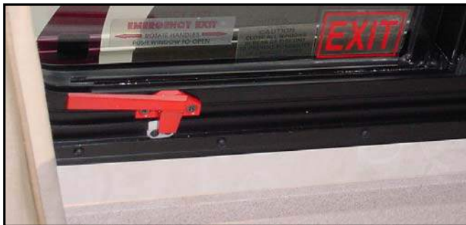
Figure 12-2. Bedroom Emergency Exit Window
