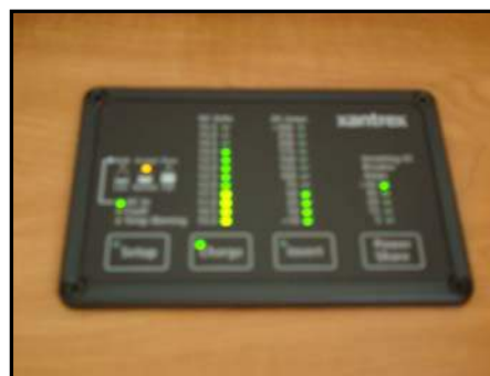
Figure 7-13. Inverter Control Panel
