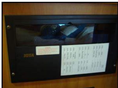
Figure 7-1. Circuit Breaker Box
