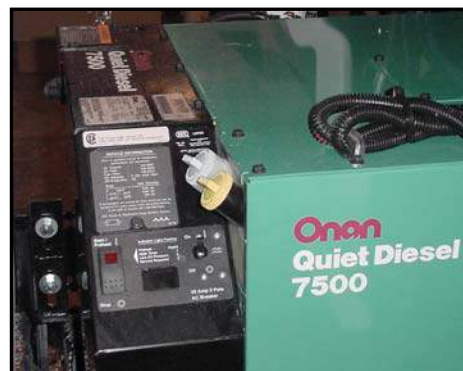
Figure 7-14. Optional Electrical Generator
