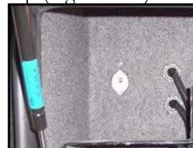
Figure 4-15. Cable & Telephone Jack
