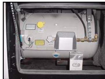
Figure 2-5. Liquid Propane Tank
