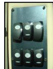
Figure 9-7. Entrance Step Switch (right middle)
