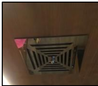
Figure 3-3: Return Air Vent
