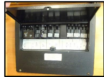
Figure 9-3: Circuit Breaker Boxes
