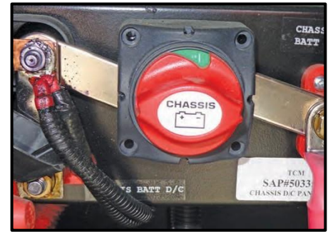
Figure 9-15: Engine Battery Disconnect Switch
