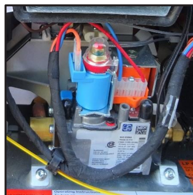
Figure 5-9: Water Heater Relief Valve
