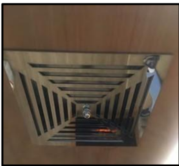
Figure 3-2: Outgoing Air Vent
