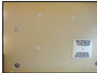
Figure 3-3: Supply Vents and A/C Unit
