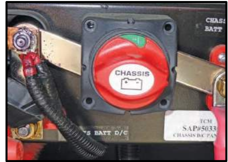
Figure 9-16: Engine Battery Disconnect Switch
