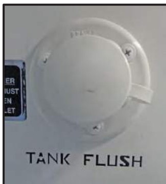
Figure 13-12: Tank Flush Connection
