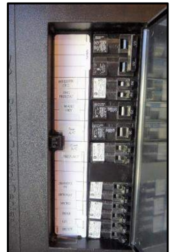
Figure 9-4: Circuit Breaker Boxes
