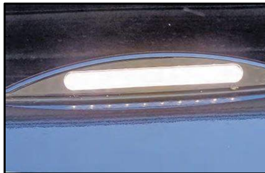
Figure 11-3: Exterior Security Light
