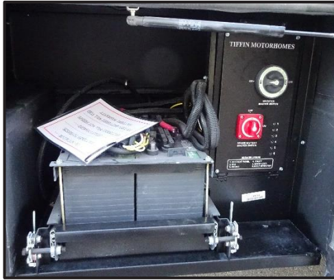
Figure 9-12: House Battery Disconnect Switch
