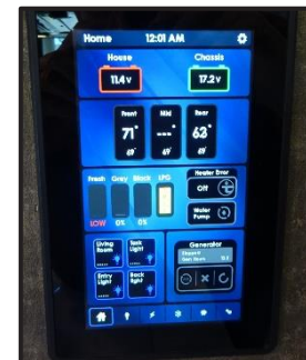
Figure 9-16: Multiplex System Switch Panel
