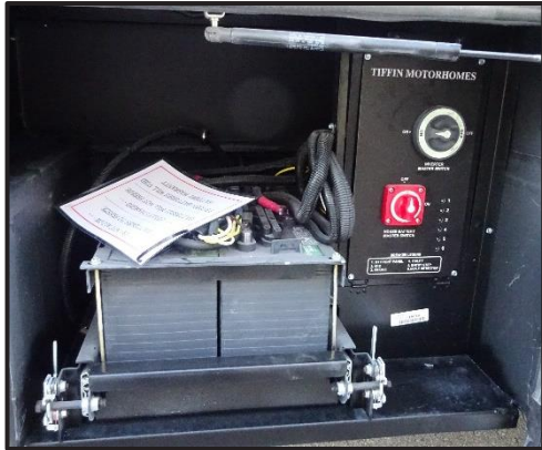
Figure 9-13: House Battery Disconnect Switch
