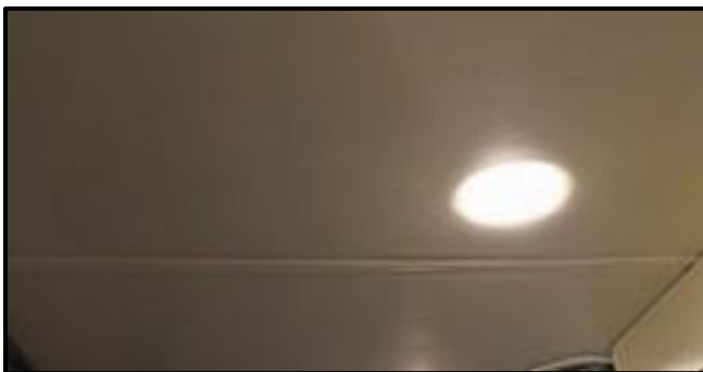
Figure 12-3: Typical Ceiling in the Allegro
