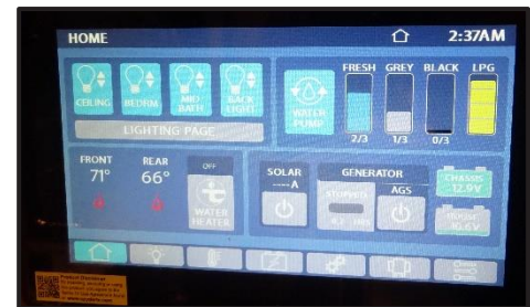
Figure 9-17: Multiplex System Switch Panel
