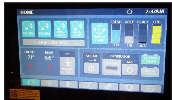
Figure 9-15: Spyder Controls Multiplexing System
