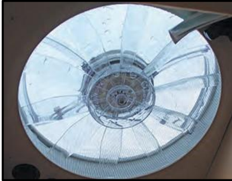
Figure 14-3: Overhead Vent Fan
