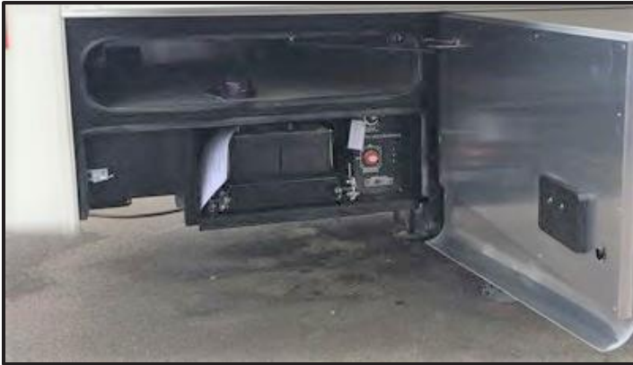
Figure 9-12: House Battery Disconnect Switch
