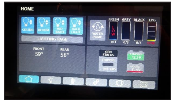
Figure 9-15: Spyder Controls Multiplexing System
