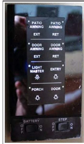
Figure 9-15: 12 VDC disconnect switch
