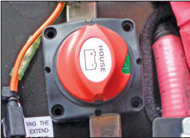
Figure 9-13: House battery disconnect switch
