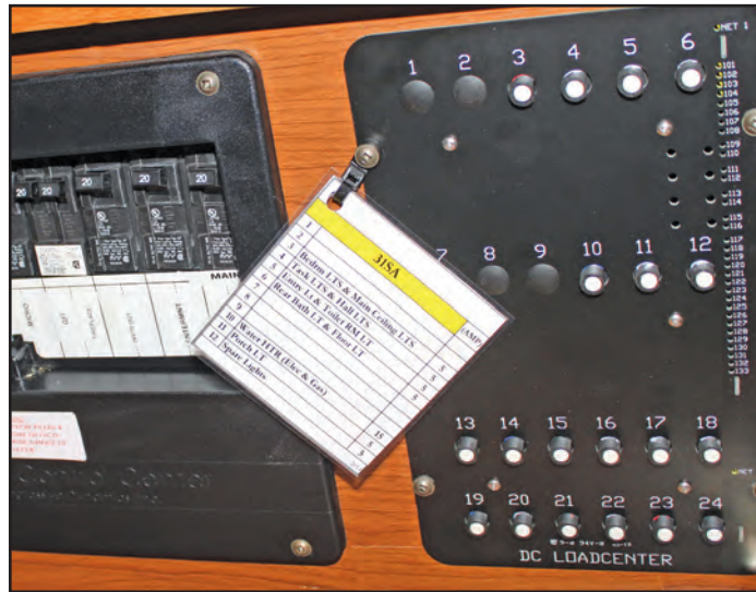
Figure 9-1: Circuit breaker box
