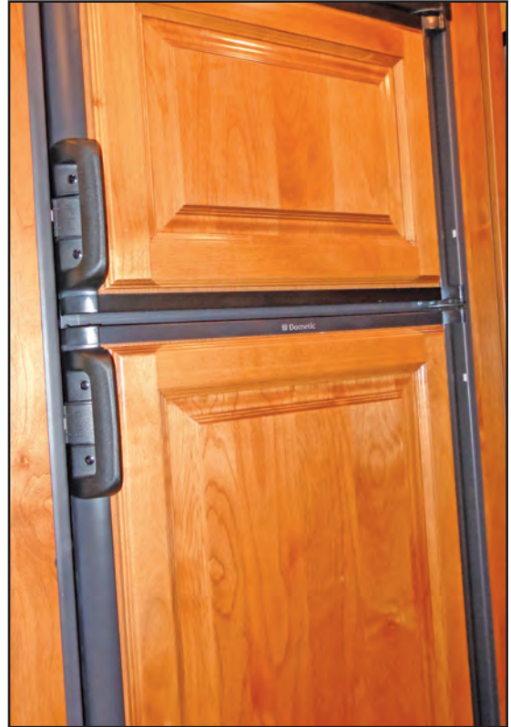
Figure 5-1: Standard LP/ Gas Refrigerator
