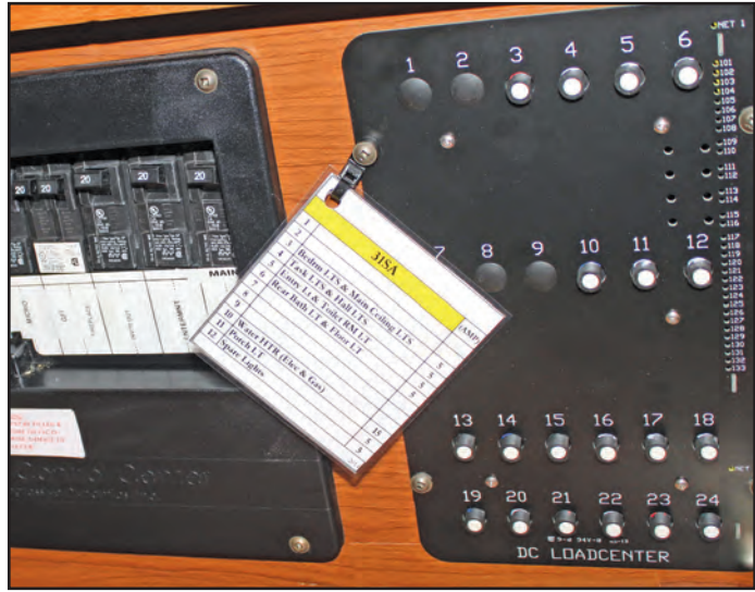
Figure 9-1: Circuit breaker box
