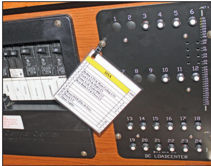
Figure 9-1: Circuit breaker box
