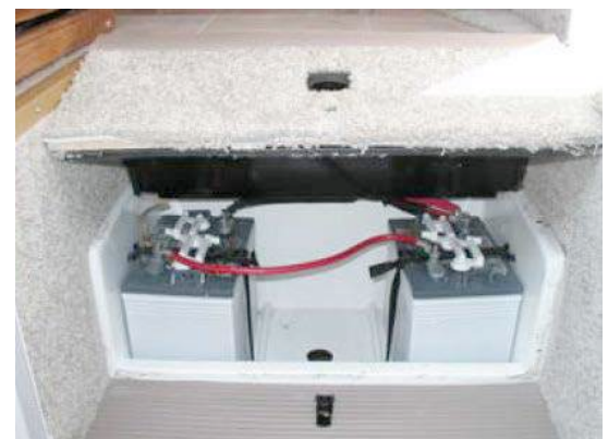
Figure 7-3. Stairwell (Top) and Battery Storage Underneath (Bottom)
