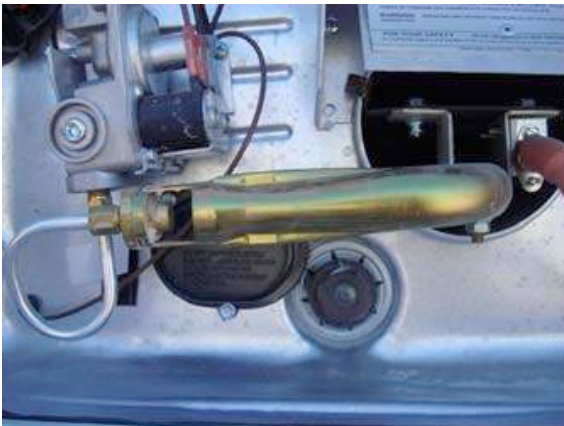
Figure 4-13. Water Heater Drain
