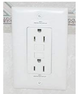
Figure 7-5. Typical AC Receptacle
