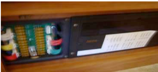
Figure 7-1. Circuit Breaker Box
