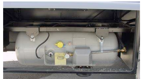
Figure 2-4. Liquid Propane Tank
