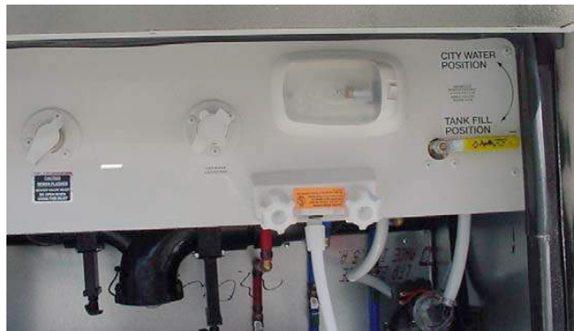
Figure 11-6. City Water Connection
