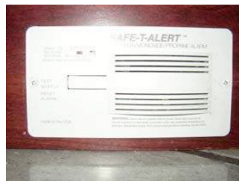
Figure 3-4. CO/LP Gas Detector
