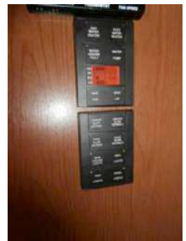
Figure 7-4. Battery Disconnect Panel
