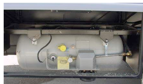
Figure 3-5. Liquid Propane Tank
