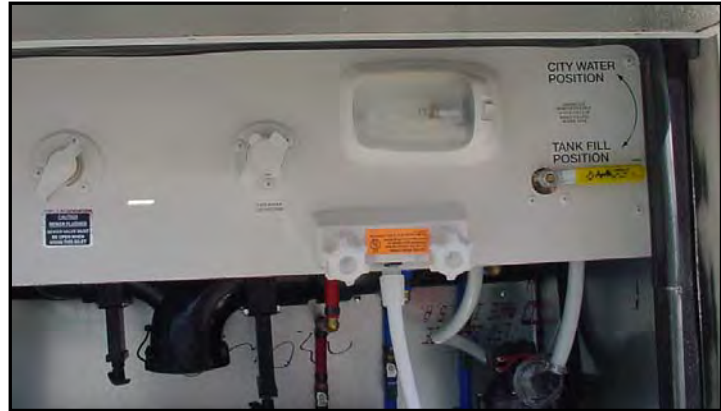
Figure 11-6. City Water Connection
