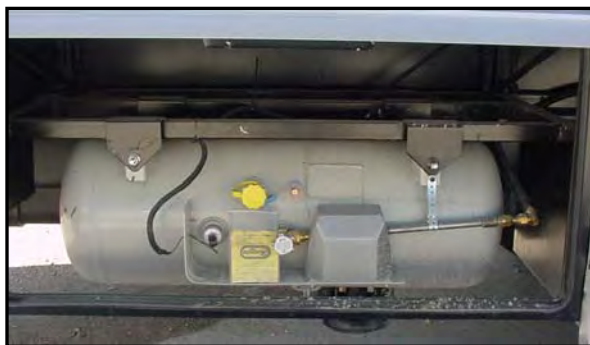
Figure 2-4. Liquid Propane Tank
