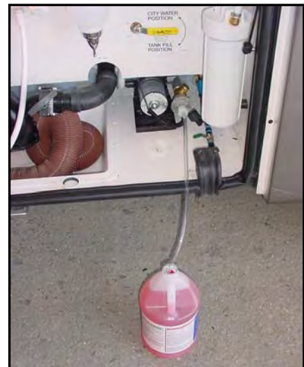
Figure 13-17. Wintering Process for the Motor Home
