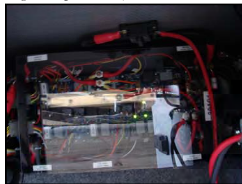
Figure 7-10. Resettable Circuit Breakers
