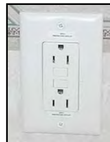
Figure 7-5. Typical AC Receptacle
