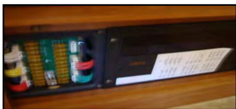
Figure 7-1. Circuit Breaker Box
