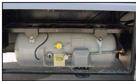
Figure 3-5. Liquid Propane Tank
