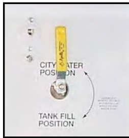
Figure 11-7. Water Fill Valve
