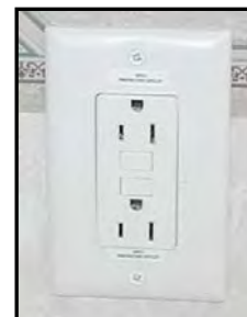
Figure 7-5. Typical AC Receptacle
