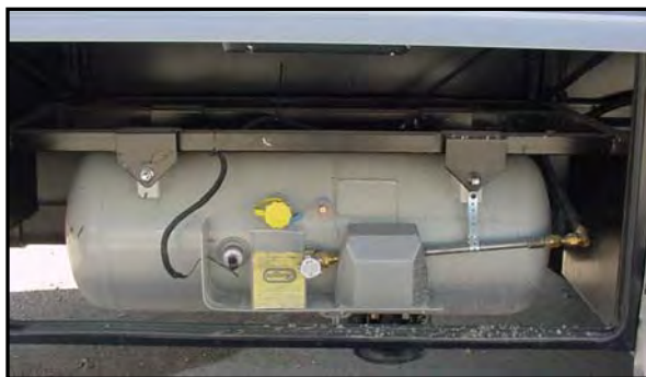
Figure 2-4. Liquid Propane Tank
