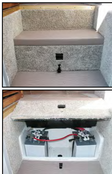
Figure 7-3. Stairwell (Top) and Battery Storage Underneath (Bottom)
