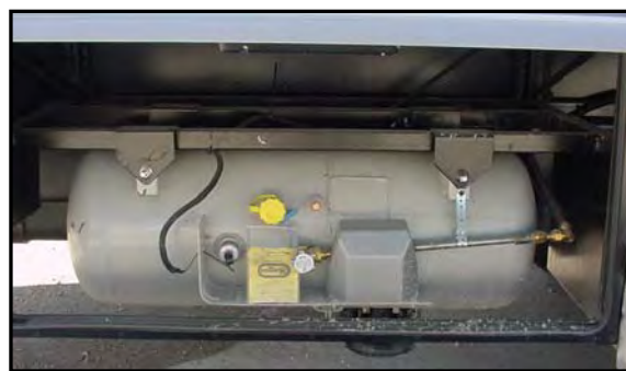
Figure 3-5. Liquid Propane Tank
