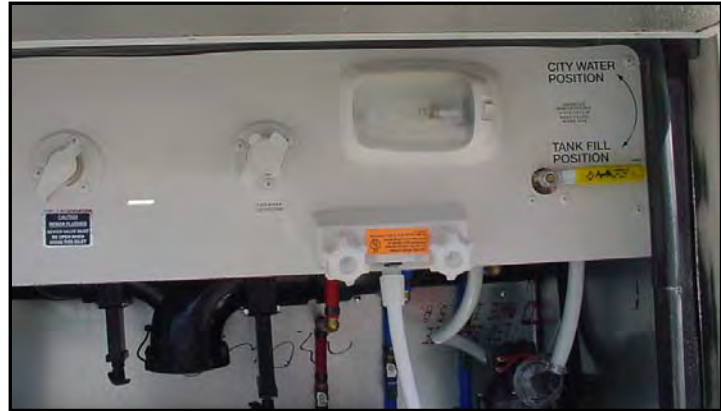
Figure 11-6. City Water Connection
