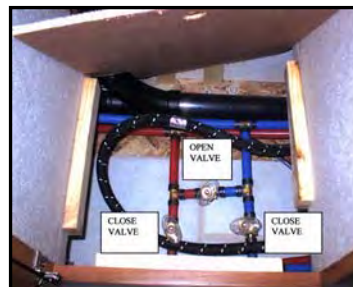
Figure 4-11. Water Heater Drain
