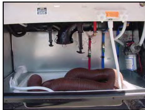
Figure 11-10. Wastewater Drain Hose and Connection in Sanitation Compartment
