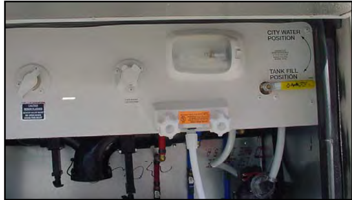
Figure 11-6. City Water Connection
