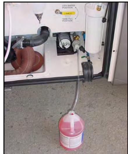
Figure 14-17. Wintering Process for the Motor Home
