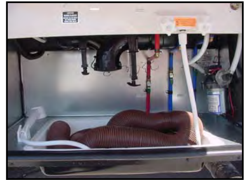
Figure 11-11. Exterior Shower in Outside Sanitation Compartment
