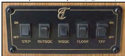
Figure 7-4. Battery Disconnect Panel
