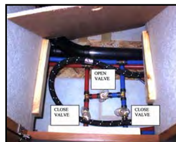
Figure 4-15. Water Heater Drain
