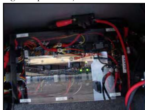
Figure 7-9. Resettable Circuit Breakers
