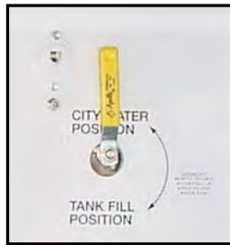
Figure 11-7. Water Fill Valve
