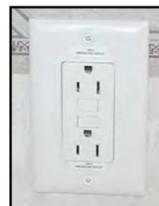
Figure 7-5. Typical AC Receptacle
