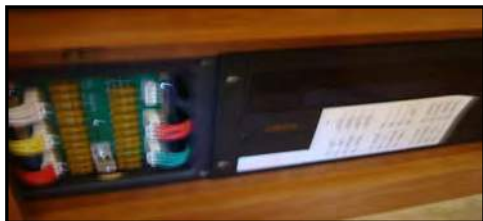
Figure 7-1. Circuit Breaker Box
