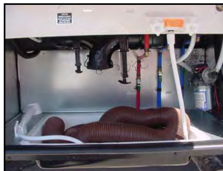
Figure 11-11. Exterior Shower in Outside Sanitation Compartment
