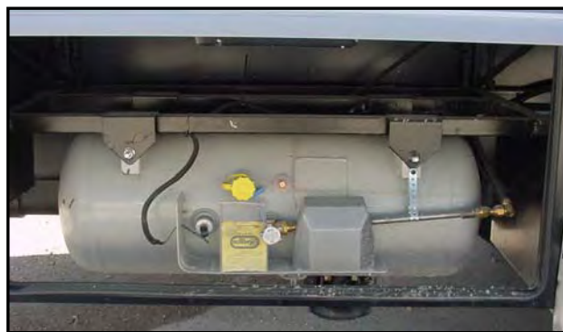
Figure 3-4. Liquid Propane Tank
