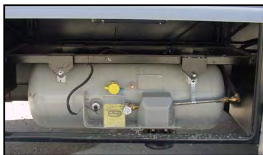
Figure 2-2. Liquid Propane Tank
