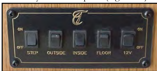
Figure 7-4. Battery Disconnect Panel
