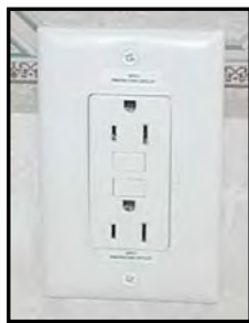
Figure 7-5. Typical AC Receptacle
