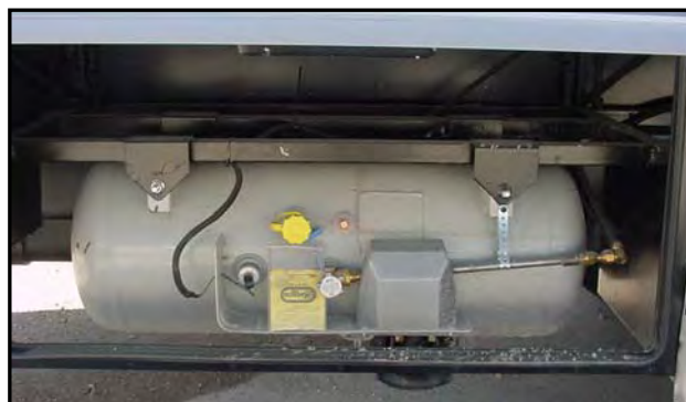
Figure 3-4. Liquid Propane Tank
