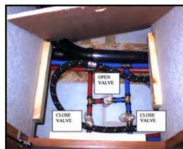
Figure 4-13. Water Heater Drain
