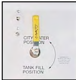
Figure 11-7. Water Fill Valve
