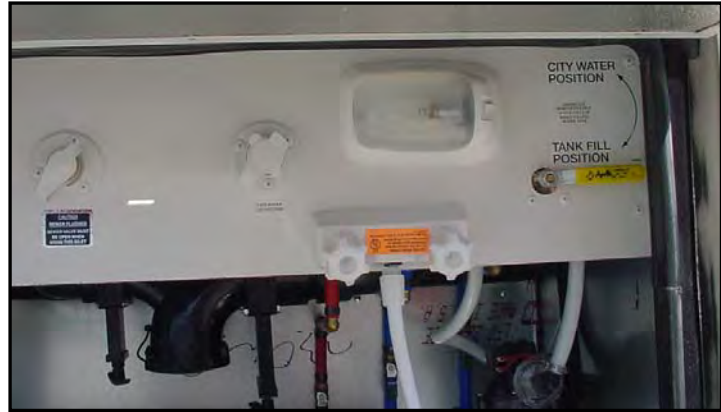
Figure 11-6. City Water Connection
