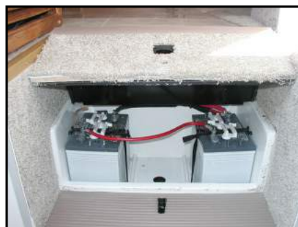
Figure 7-3. Stairwell (Top) and Battery Storage Underneath (Bottom)
