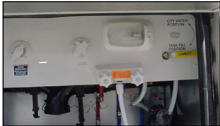
Figure 11-6. City Water Connection
