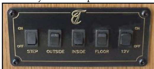
Figure 7-4. Battery Disconnect Panel
