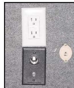
Figure 7-6. Typical 12VDC Receptacle (Bottom)
