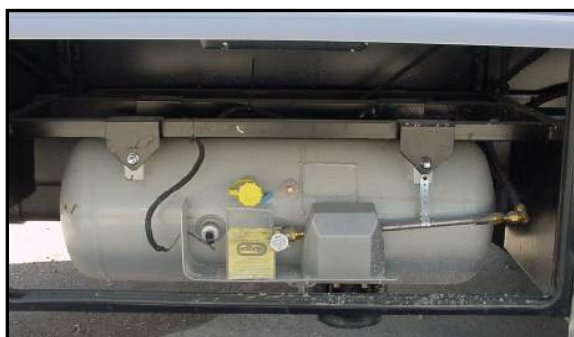
Figure 2-4. Liquid Propane Tank
