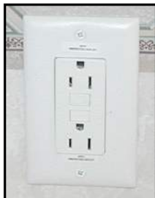
Figure 7-5. Typical AC Receptacle
