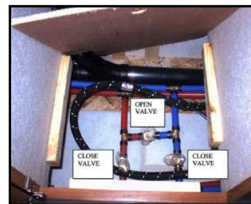
Figure 4-13. Water Heater Drain
