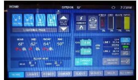
Figure 3-2: Home Screen for the Spyder Controls System
