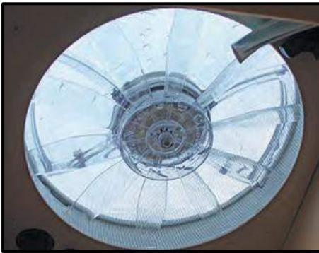
Figure 14-5: Overhead Vent Fan
