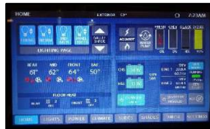
Figure 13-7: Spider Controls System Switch
