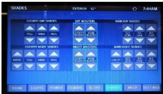
Figure 12-11: Day/Night Window Shade Control
