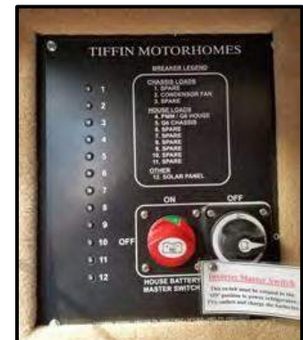
Figure 9-4: House Battery Disconnect Panel Switch
