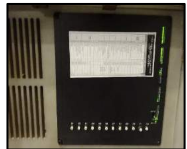
Figure 9-1: Circuit Breaker Box
