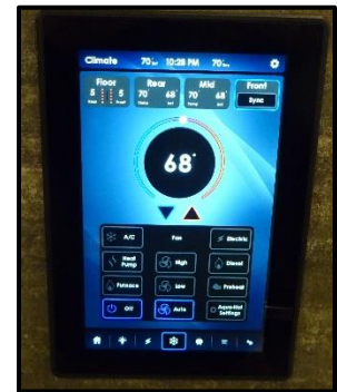
Figure 0-7: Heat Pump Controls
