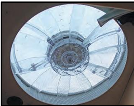
Figure 0-3: Overhead Vent Fan
