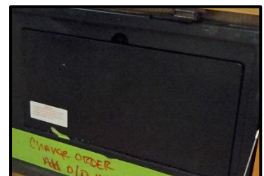
Figure 0-1: Circuit Breaker Box
