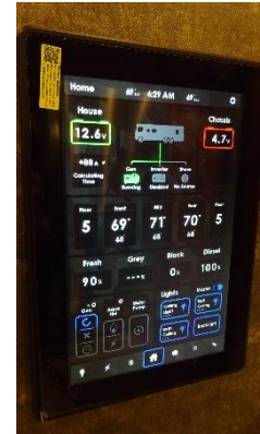
Figure 3-2: Home Screen for the Spyder Controls System
