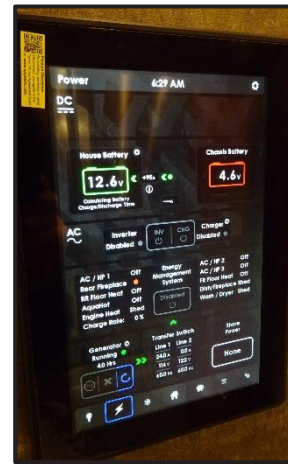
Figure 9-12: Energy Management System
