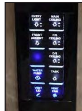
Figure 13-7: Water Pump Switch
