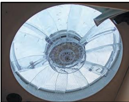
Figure 14-5: Overhead Vent Fan
