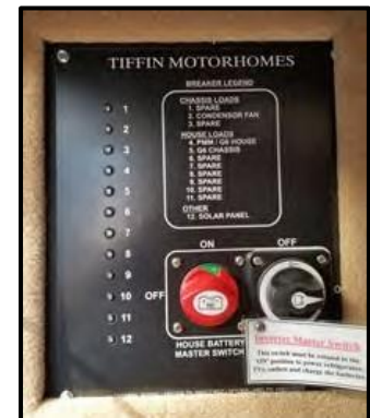
Figure 9-4: House Battery Disconnect Panel Switch
