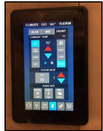
Figure 4-7: Heat Pump Controls
