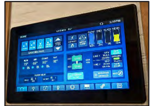
Figure 3-2: Home Screen for the Spyder Controls System
