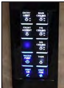
Figure 13-6: Water Pump Switch
