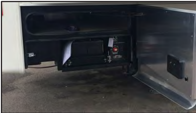
Figure 9-5: House Battery Disconnect Switch Location
