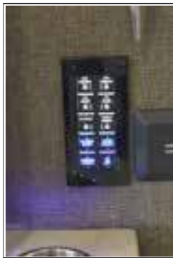
Figure 5-7 : Television lift control panel located in the living room slide out box.
