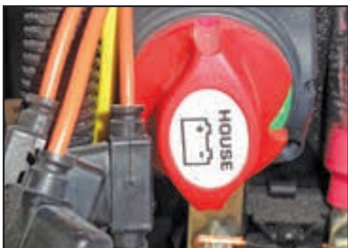
Figure 8-4: House battery disconnect panel switch
