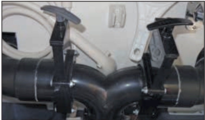
Figure 12-10: Sanitation coupling, valve and hose
