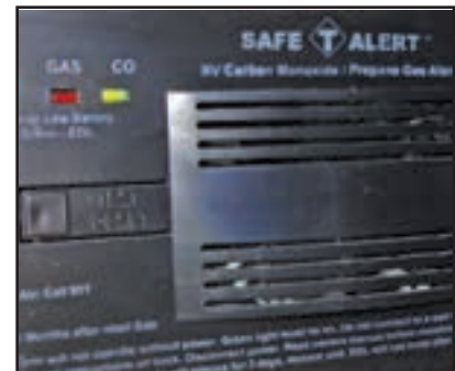
Figure 2-5: Carbon Monoxide alarm
