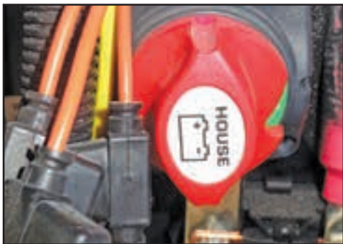
Figure 8-4: House battery disconnect panel switch
