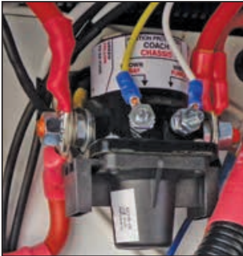
Figure 8-6: 12 VDC disconnect switch
