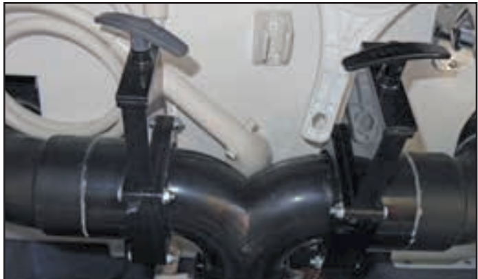
Figure 12-10: Sanitation coupling, valve and hose
