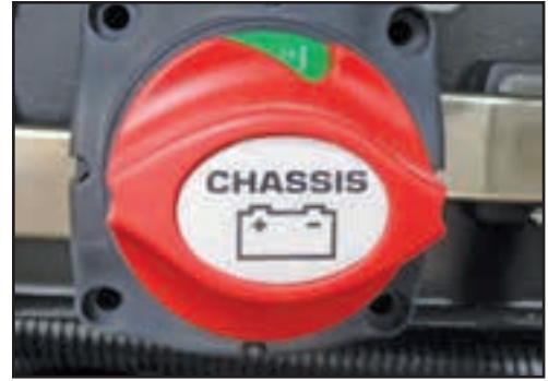
Figure 8-5: Engine battery disconnect panel switch
