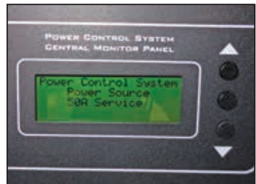
Figure 8-13: Energy management system
