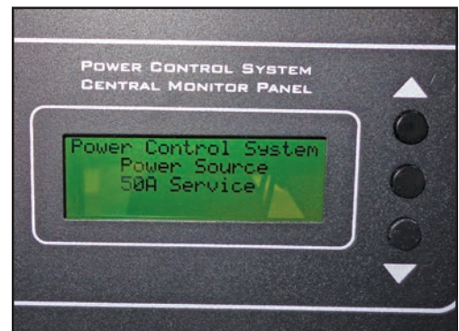
Figure 8-13: Energy management system
