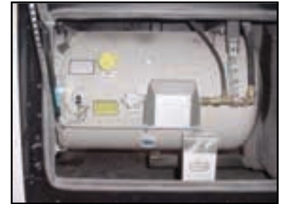
Figure 2-3. Liquid Propane Tank
