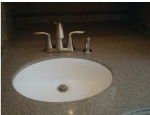
Figure 11-3. Bathroom Sink and Faucet
