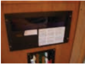
Figure 7-1. Circuit Breaker Box
