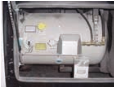
Figure 3-7. Liquid Propane Tank
