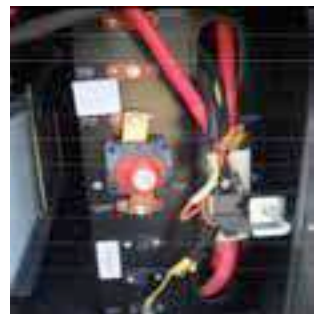
Figure 7-9. Rotary Switch to Disconnect “House” Batteries
