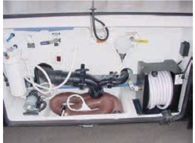
Figure 11-13. Exterior Shower in Outside Compartment
