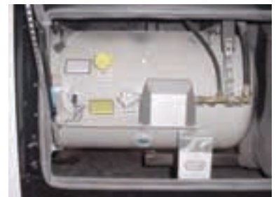
Figure 2-4. Liquid Propane Tank
