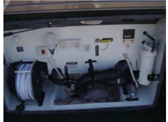
Figure 11-11. Sanitation Compartment Containing Holding Tank Drains and Flexible Drain Hose
