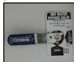
Figure 11-10. Water Heater Bypass
