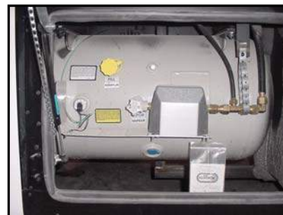
Figure 2-4. Liquid Propane Tank
