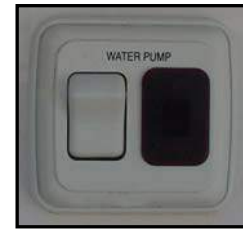
Figure 11-6. Water Pump Switch
