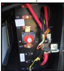
Figure 7-8. Rotary Switch to Disconnect Engine Battery
