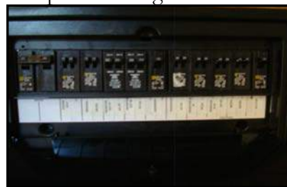
Figure 7-16. Energy Management System
