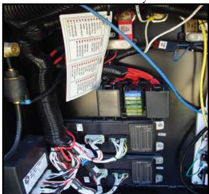
Figure 7-2. 12 VDC Fuse Panels
