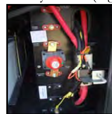
Figure 7-9. Rotary Switch to Disconnect “House” Batteries
