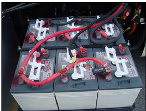
Figure 7-5. 12 VDC Battery Supply (Compartment)
