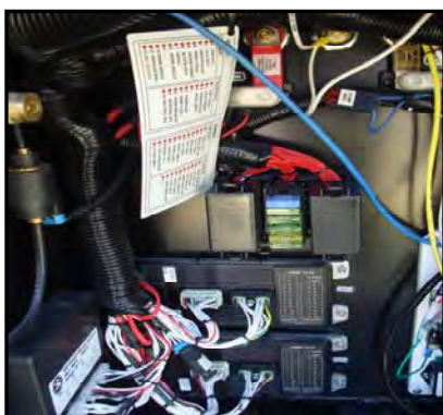
Figure 7-2. 12 VDC Fuse Panels
