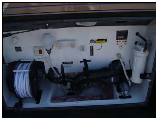
Figure 11-13. Sanitation Compartment Containing Holding Tank Drains and Flexible Drain Hose
