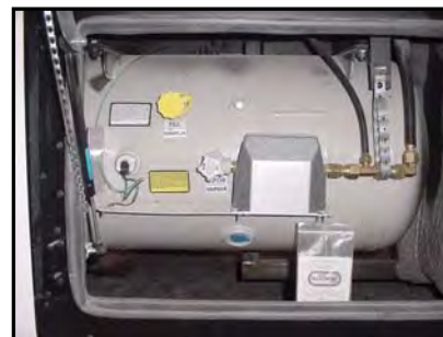
Figure 2-4. Liquid Propane Tank
