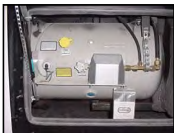
Figure 3-7 Liquid Propane Tank
