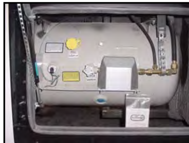
Figure 2-3. Liquid Propane Tank
