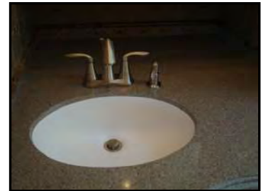
Figure 11-3. Bathroom Sink and Faucet
