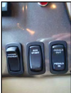
Figure 7-3. Auxiliary Start Switch (Center)
