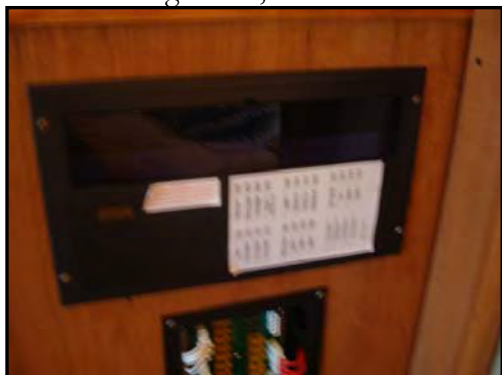
Figure 7-1. Circuit Breaker Box
