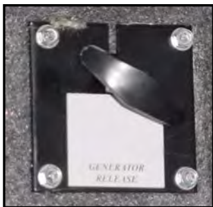
Figure 7-18. “Pull” Cable for Generator Release
