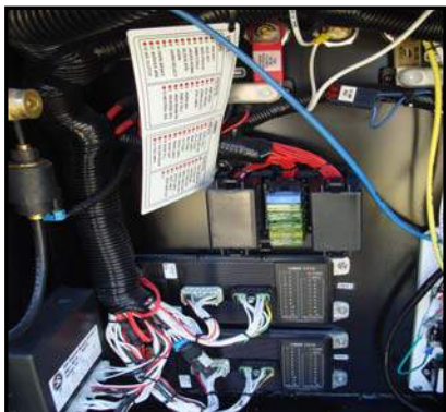
Figure 7-2. 12 VDC Fuse Panels
