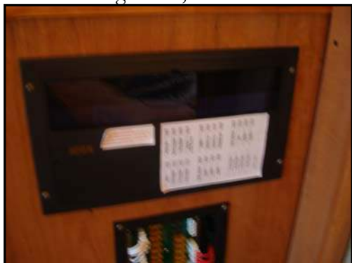
Figure 7-1. Circuit Breaker Box
