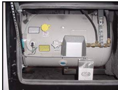
Figure 2-3. Liquid Propane Tank
