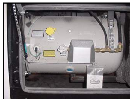
Figure 2-4. Liquid Propane Tank
