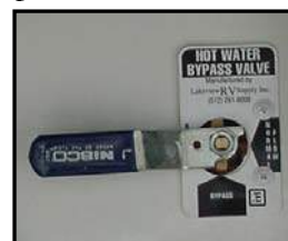
Figure 11-10. Water Heater Bypass
