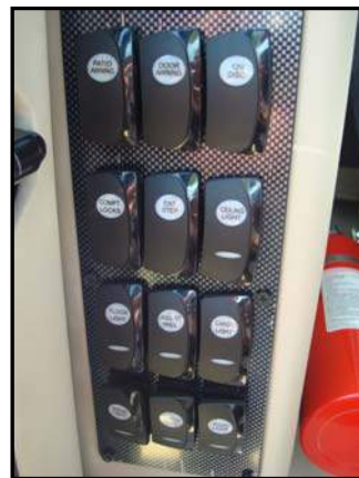
Figure 7-10. 12 VDC Disconnect Switch
