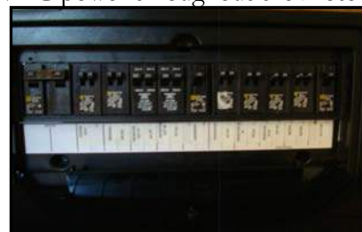
Figure 7-15. Energy Management System
