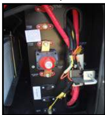
Figure 7-8. Rotary Switch to Disconnect Engine Battery
