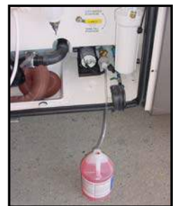
Figure 14-16. Winterizing the Water System
