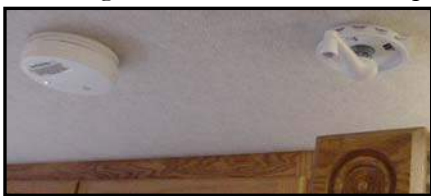
Figure 2-6. Smoke Detector (Left)
