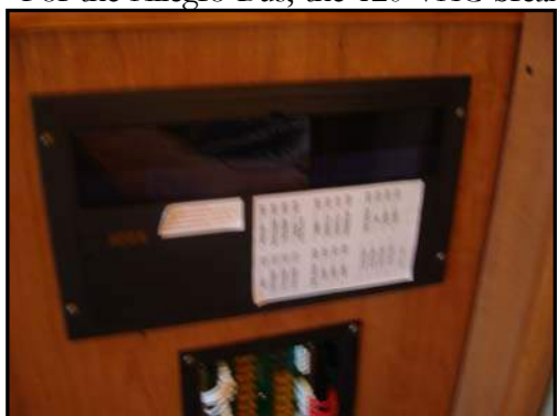
Figure 7-1. Circuit Breaker Box
