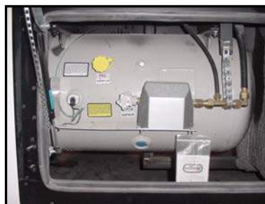
Figure 2-4. Liquid Propane Tank
