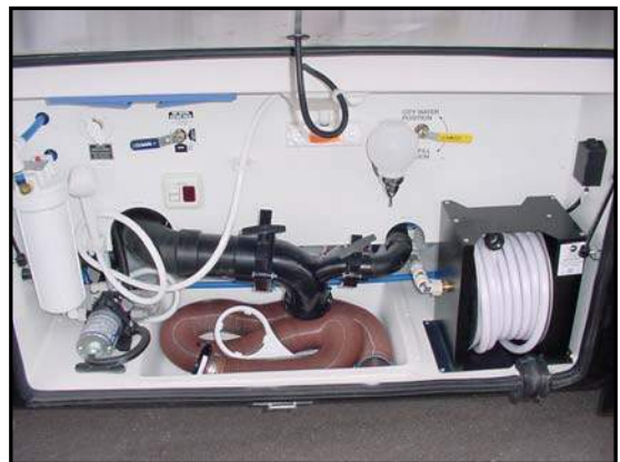
Figure 11-15. Exterior Shower in Outside Compartment
