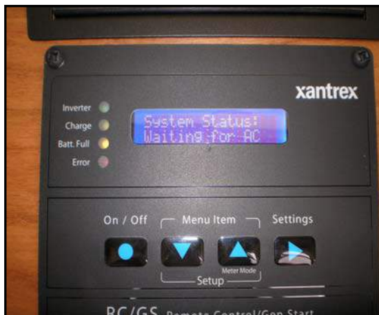
Figure 7-15. Inverter Control Panel
