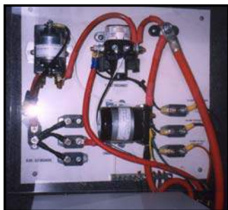
Figure 7-18. Resettable Circuit Breakers
