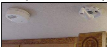
Figure 2-7. Smoke Detector (Left)
