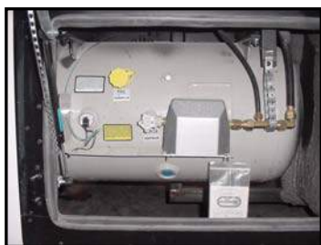
Figure 3-7 Liquid Propane Tank
