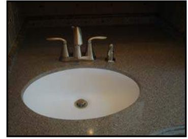
Figure 11-3. Bathroom Sink and Faucet
