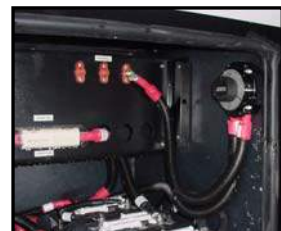
Figure 7-9. Rotary Switch to Disconnect “House” Batteries
