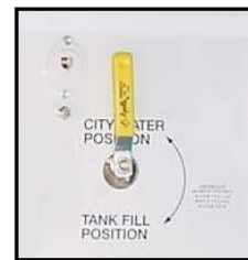
Figure 11-8. Water Fill Valve
