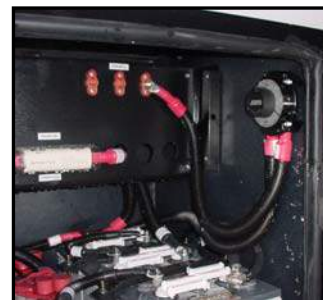
Figure 7-7. Rotary Switch to Disconnect “House” Batteries
