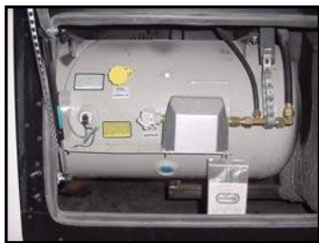
Figure 3-7 Liquid Propane Tank
