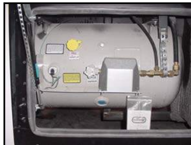
Figure 2-4. Liquid Propane Tank
