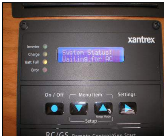
Figure 7-13. Inverter Control Panel
