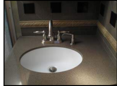
Figure 11-3. Bathroom Sink and Faucet
