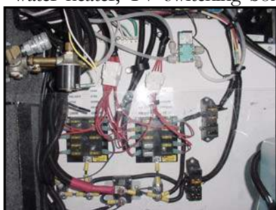
Figure 7-2. 12 VDC Fuse Panels
