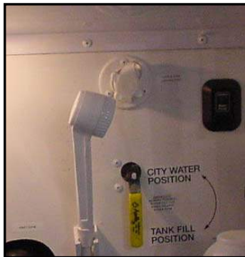
Figure 11-8. City Water Connection
