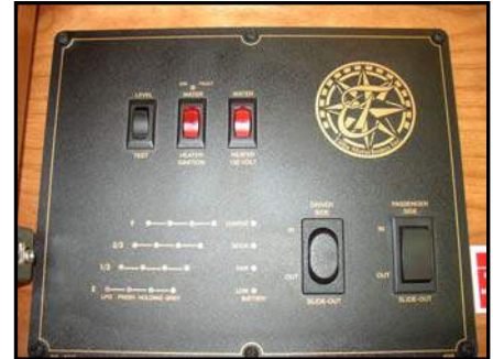
Figure 11-1. Monitor Panel (Water, LP Gas, Battery)
