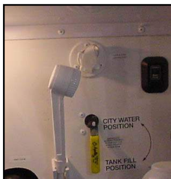
Figure 11-8. City Water Connection
