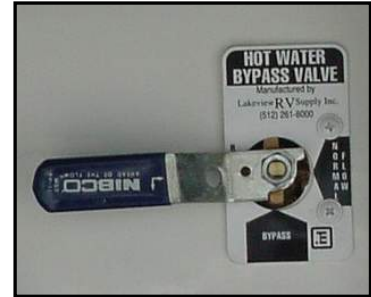
Figure 11-11. Water Heater Bypass
