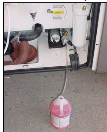
Figure 14-16. Winterizing the Water System
