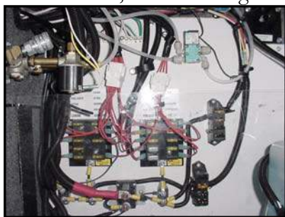
Figure 7-2. 12 VDC Fuse Panels
