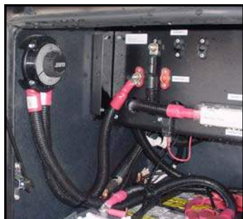
Figure 7-6. Rotary Switch to Disconnect Engine Battery
