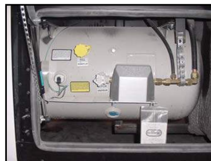
Figure 2-4. Liquid Propane Tank
