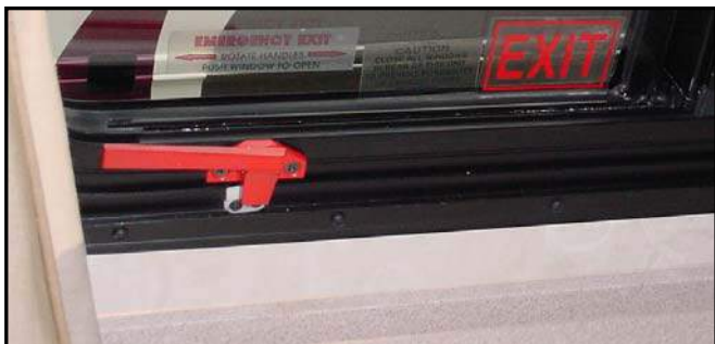
Figure 13-2. Bedroom Emergency Exit Window
