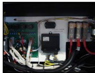
Figure 7-4. 12 VDC Battery System
