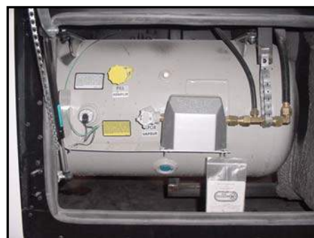
Figure 2-2. Liquid Propane Tank
