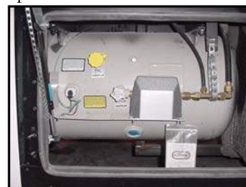
Figure 2-4. Liquid Propane Tank
