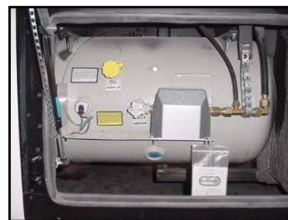
Figure 3-4. Liquid Propane Tank
