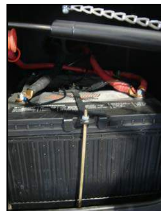
Figure 7-5. House Batteries (Underneath Entrance Door Step Well)
