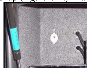
Figure 4-14. Cable & Telephone Jack
