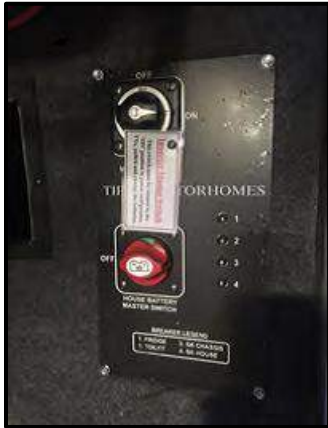
Figure 9-10: House Battery Disconnect Panel
