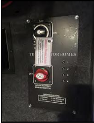
Figure 9-11: House Battery Disconnect Panel
