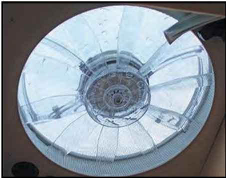
Figure 14-5: Overhead Vent Fan
