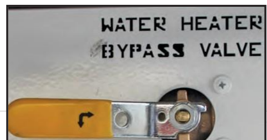
Figure 13-9: Water Heater Bypass System
