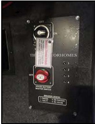
Figure 9-11: House Battery Disconnect Panel
