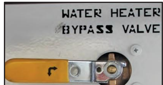
Figure 13-9: Water Heater Bypass System
