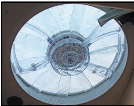
Figure 14-5: Overhead Vent Fan
