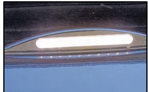
Figure 11-3: Exterior Security Light
