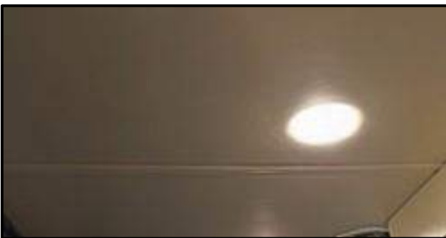
Figure 12-3: Typical Ceiling in the Allegro Breeze
