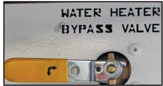
Figure 13-9: Water Heater Bypass System
