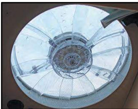
Figure 14-3: Overhead Vent Fan
