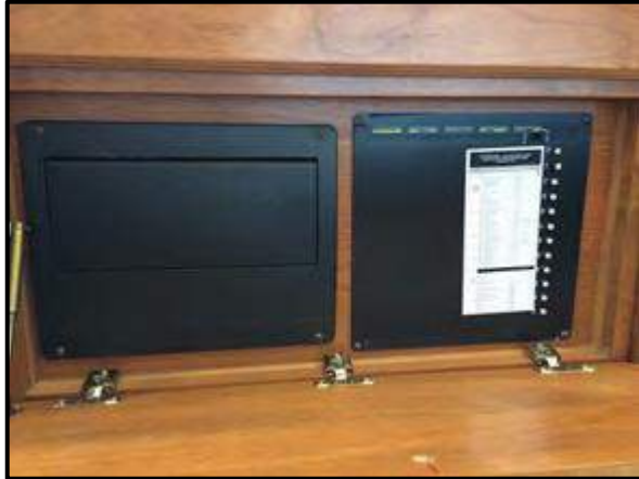
Figure 9-3: Multiplex System (Inside Circuit Breaker Box)
