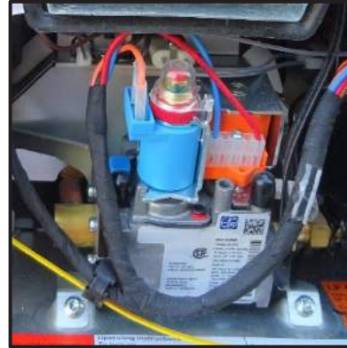
Figure 5-9: Water Heater Relief Valve
