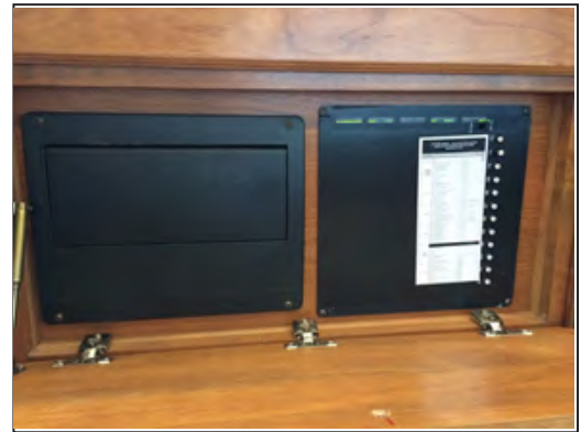
Figure 9-3A: Inside circuit breaker box
