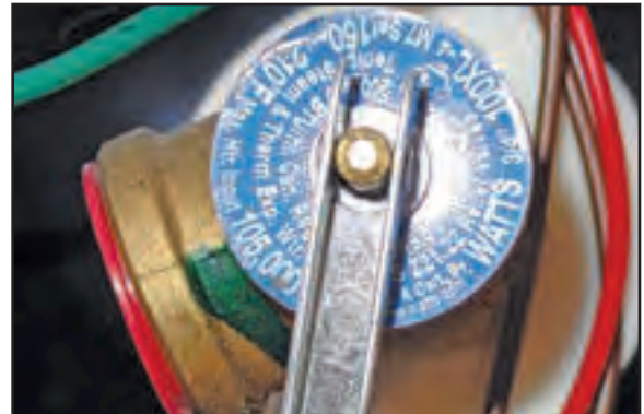
Figure 5-9: Water heater relief valve
