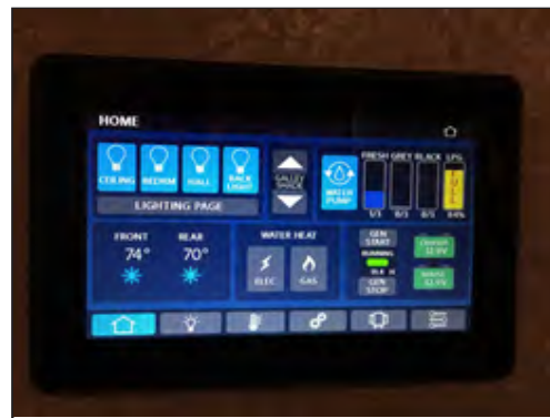
Figure 13-5: Water pump controls
