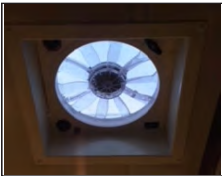
Figure 14-3: Overhead vent fan
