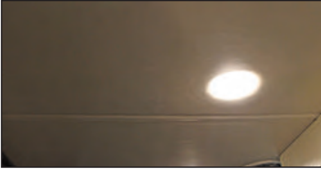
Figure 12-3: Typical ceiling in the Allegro Breeze
