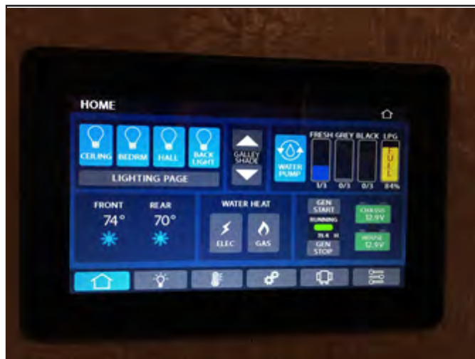
Figure 5-7: Water heater controls
