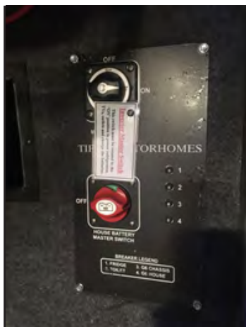
Figure 9-9: House battery disconnect panel
