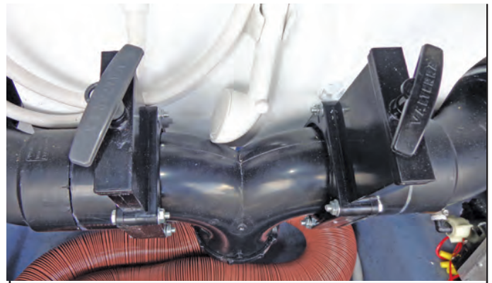
Figure 13-10: Sanitation coupling, valve and hose
