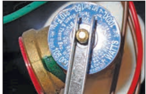
Figure 5-10: Water heater relief valve
