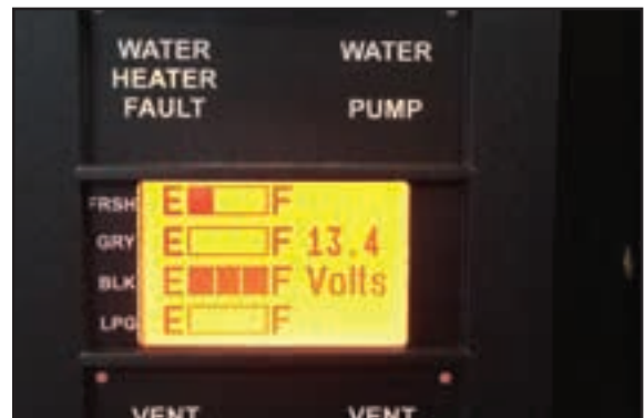
Figure 13-5: Water pump switch
