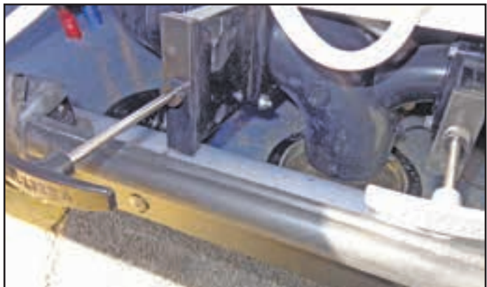
Figure 13-11: Sanitation coupling, valve and hose
