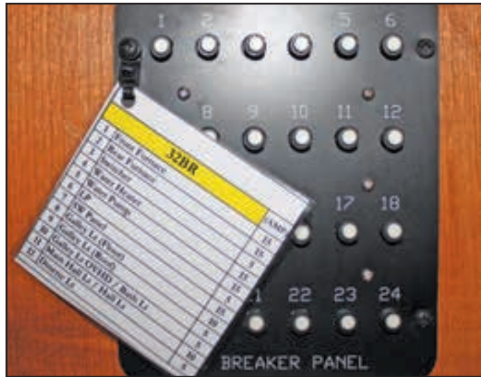
Figure 9-1: Circuit breaker box
