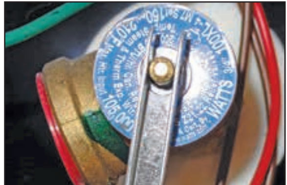
Figure 5-10: Water heater relief valve
