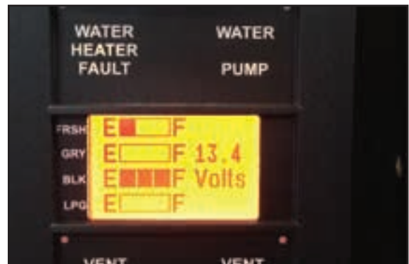
Figure 13-5: Water pump switch
