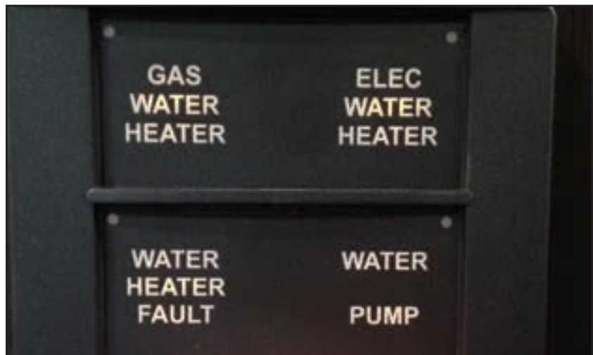
Figure 5-8: Water heater switches
